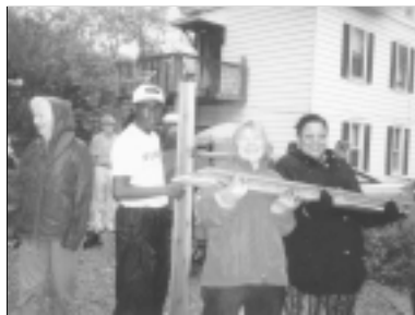
Phyllis Beck, Robin Kwizera and a youth from Shalom, carrying lumber during a building project.
