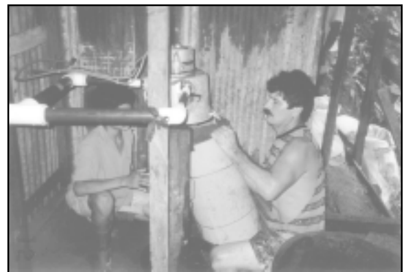
Ricardo, a capable and hospitable leader of the community, adding a splash guard to the Pelton wheel discharge
