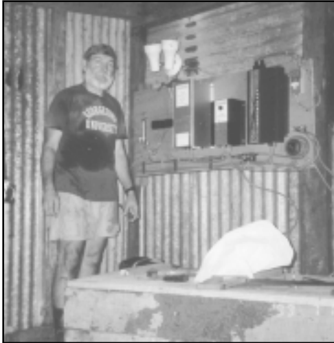
Ben Watkins, Lisle participant and volunteer, stands by the completed electric module.
