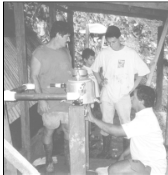
From left to right: Ricardo, Ronald, and Franklin making final adjustments for the location of the Pelton wheel.
